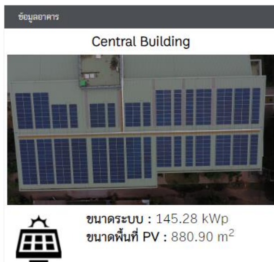
Fig.2 The details of installed the solar PV system
