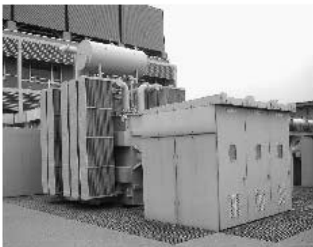
Fig. 3 Main Transformer and GIS.
