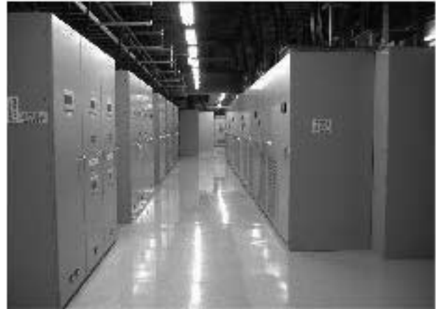
Fig. 6 MV/LV Switchgears in electrical room 2.
